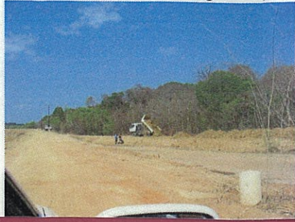
Figure 17. Oct 05. Construction of SW dike viewed SW of base camp (white PVC pipe protecting valve).
