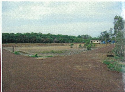
Figure 23. Nov 05. Dry road base on top of dike walls of Pond 1 (NW corner view where electrical cable will run to base camp).
