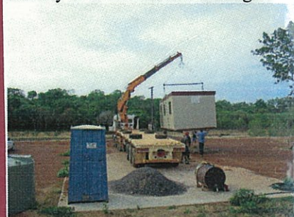
Figure 27. Nov 05. Demountable delivered to base camp and positioned directly over foundation footings.
