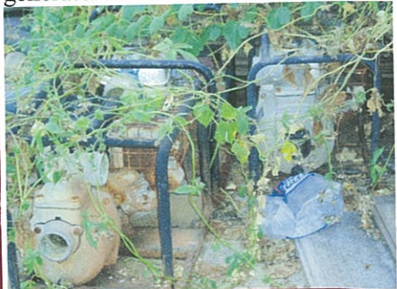
Figure 41. Abandoned generators at the crab farm.
