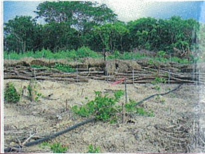
Figure 35. Nov 05 soil stabilisation with black poly pipe freshwater line (note mangrove regrowth).
