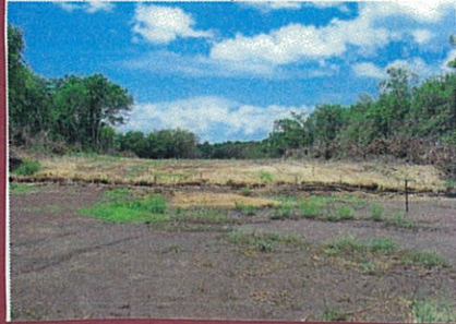
Figure 36. Oct 05. Soil stabilisation of easement on Dickward Drive side of Farm (frontal view).
