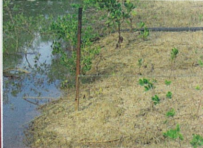
Figure 38. Nov 05. Rope 100mm above cleared topsoil stretched between stakes to measure the occurrence of erosion along foreshore of saltwater tidal creek (note black poly water pipe).
