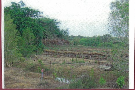
Figure 34. Oct 05. East view of easement showing soil stabilisation structures made of hay/coffee bush logs.
