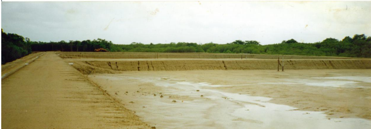
Above: Excavations for the Kulaluk prawn farm aquaculture project on the old salt pan in 1997.
