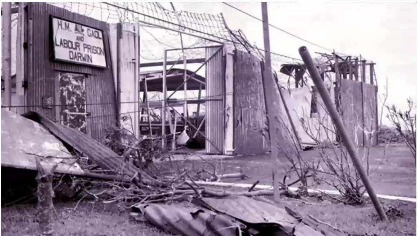
Two photographs from the NT Library collection of damage done to Fannie Bay Gaol by Cyclone Tracy on Christmas Day, 1974. Fred Fogarty had been sentenced to 12 months a few months earlier.
