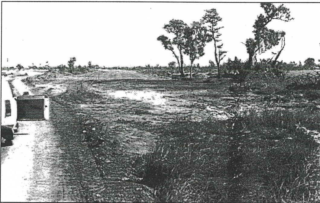
Photograph Twelve: Work on the 'Connector Road', later called Dick Ward Drive, begins, August 1979 (Northern Territory Archives, WB Day Collection NTRS 75 Photo 78)
